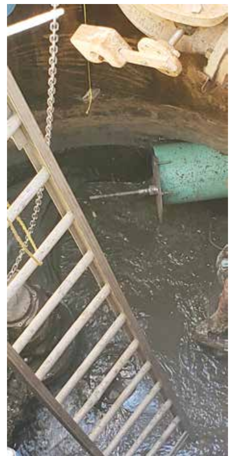
Installed 750mm pipe section with ready rod 'clamp'. Note 'awkward' position of pipe entering pump station
